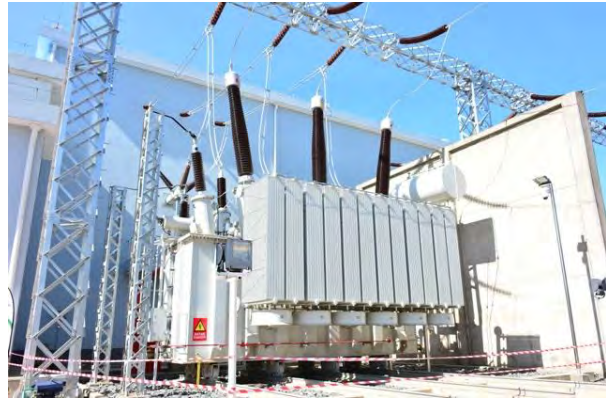
Figure 6-17 Existing GIS 2x200MVA Substation
