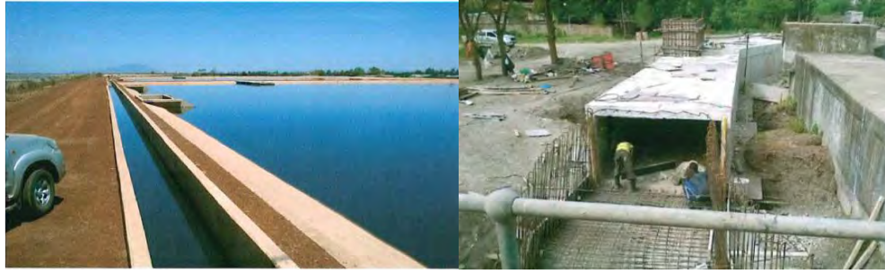
Figure 4-50 Dandora Sewerage Treatment Plant and Dandora Trunk Sewer
