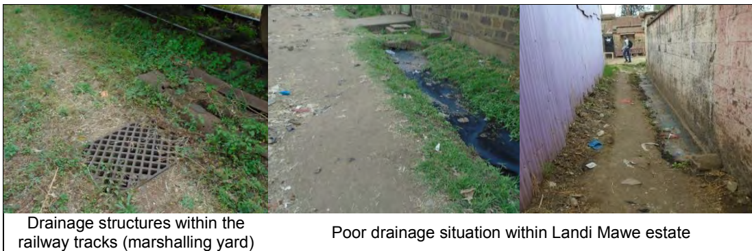
Figure 4-20 State of Drainage in the Planning Area
